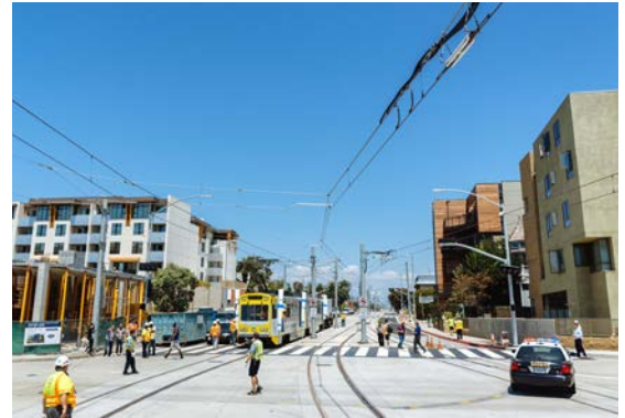
Trained flaggers ensure the safe crossing of pedestrians and workers of an adjacent development.
