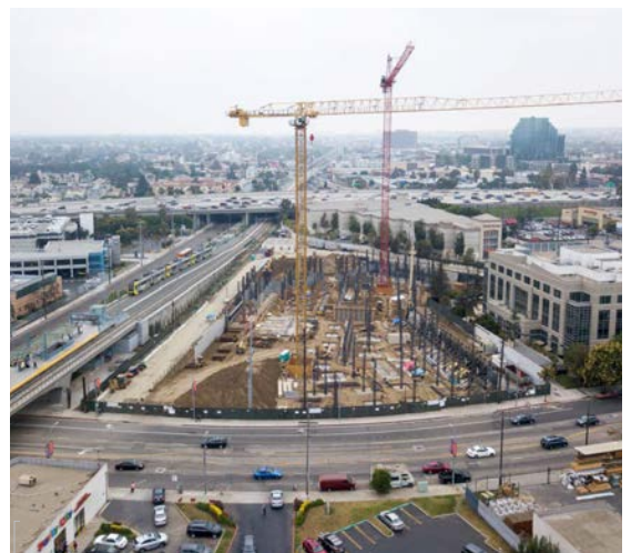
Construction adjacent to the active ROW may require ongoing coordination with Metro.
